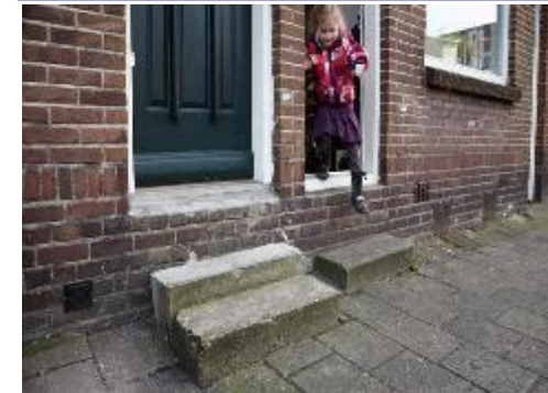
Damage through soil subsidence
